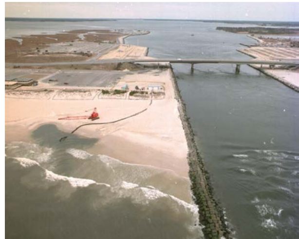
Figure 7 Crane-mounted mobile jet pump sand bypass system – Indian River Inlet, Delaware (Source: [7])
